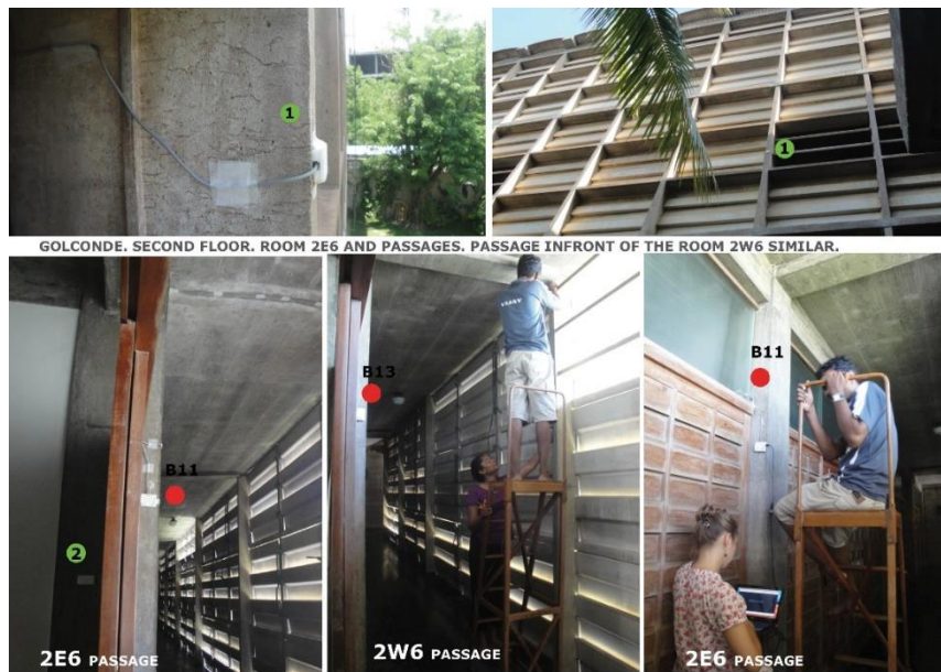
Figure 17 Placement of loggers on the Second Floor - East and West passages
